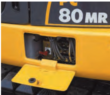
The battery main switch is standard
